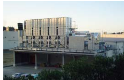
Effluent gas treatment equipment (Fukuoka Plant)
